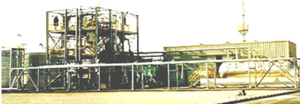
10 TPD HEXAMINE PLANT
